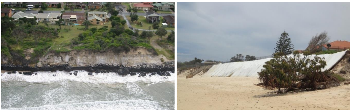
Figure 2 Impacts of shoreline recession at Lake Cathie Beach (left) and Old Bar Beach (right), including shoreline encroachment and loss of beach amenity. Photos: OEH/M Kinsela, OEH.
